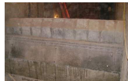
METAL-ROK® cricket wall shapes installed with TUFF-FLO® 47 cast underneath within the steel support
